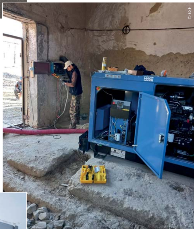
Generator installed in a Moldovan hospital by Electricians Without Borders
